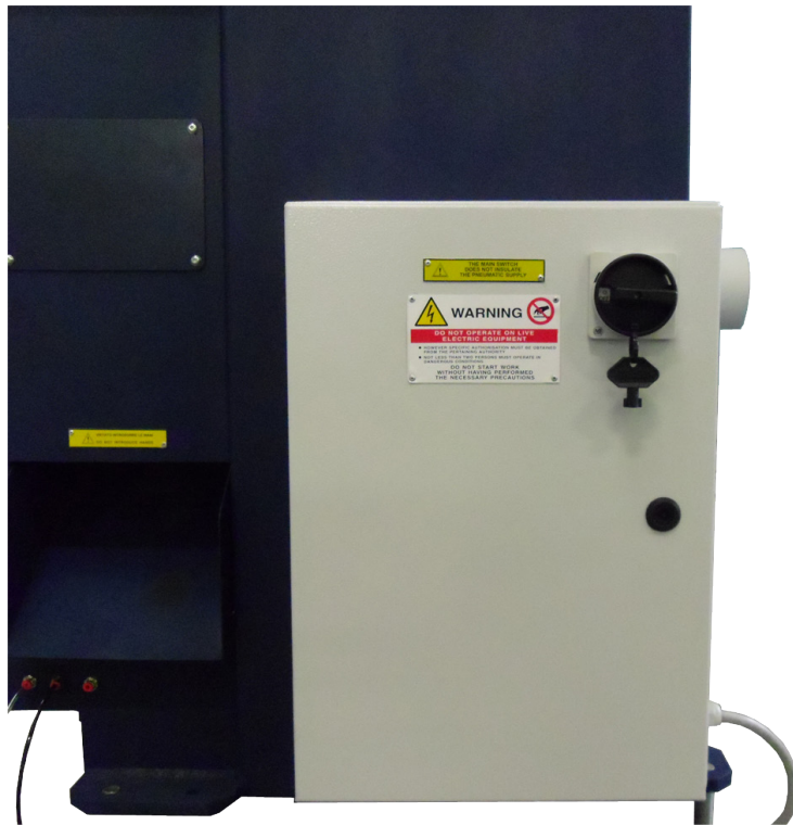
Picture 4.6.2 A – Electric Panel Disposition
